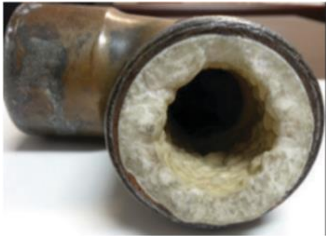
Hard water build up in feedwater pipe—had to be replaced and serviced regularly at $15,000/yr
