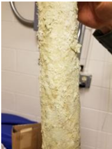
Scale build-up on inline filters that were not properly serviced
