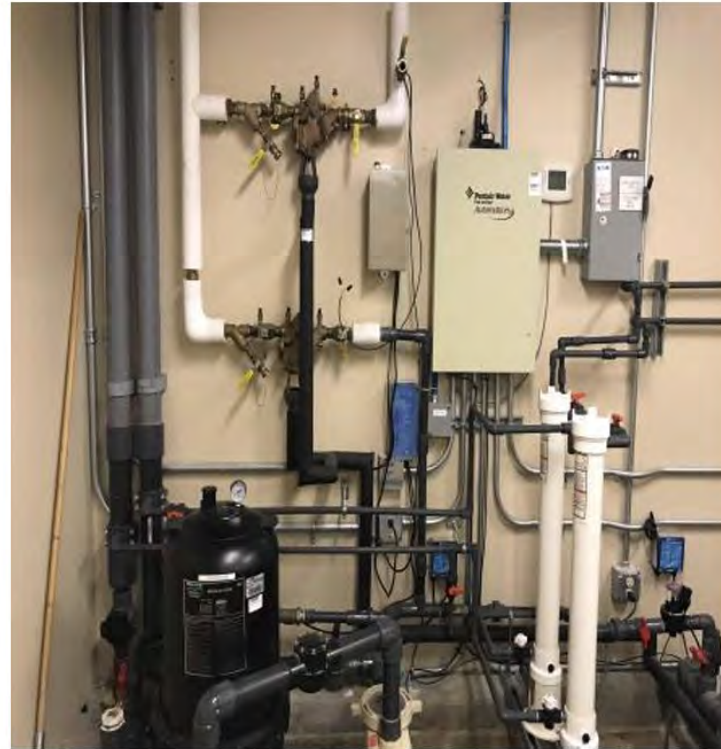
RPBP-Supplies to Irrigation System and Dec. Fountain.
